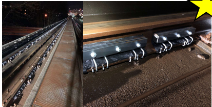
Rail Dampers (hotspots)
