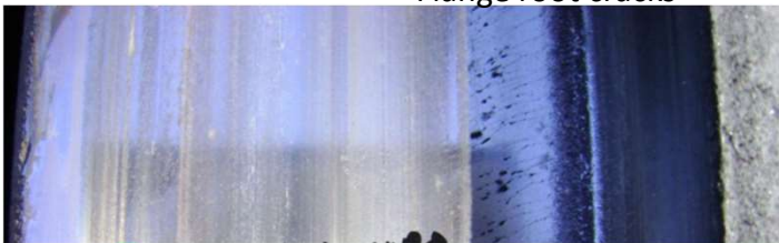
Flange root cracks
