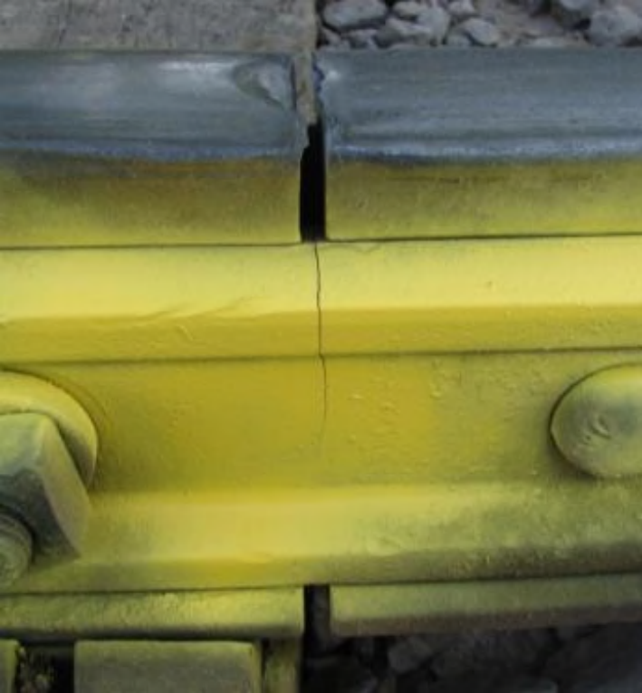
Cracked/Broken Joint Bar
