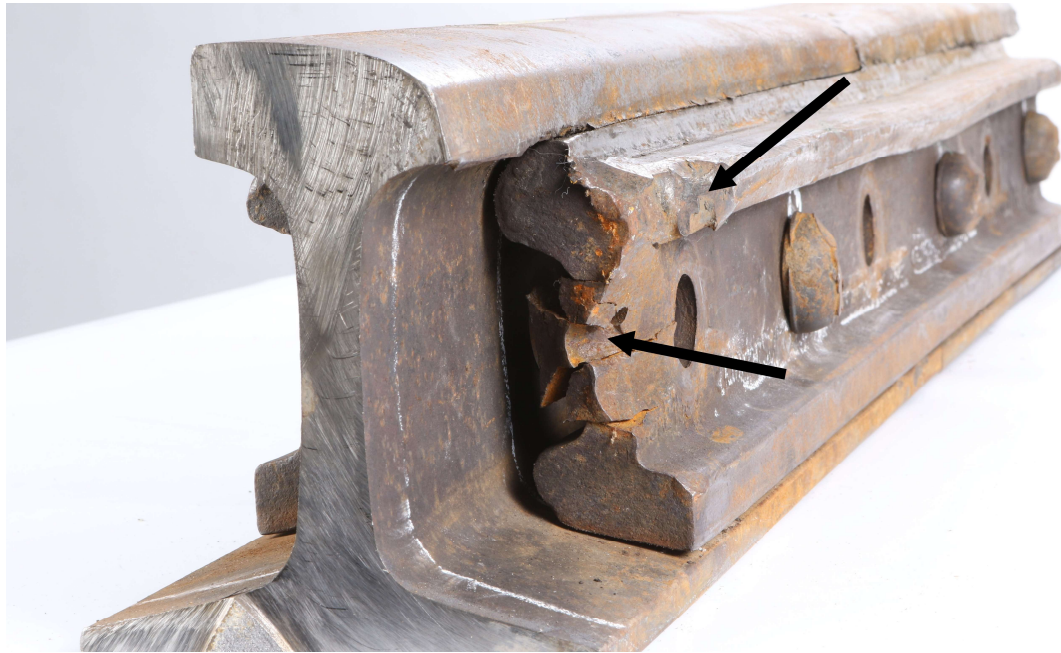
South plug rail joint bar
